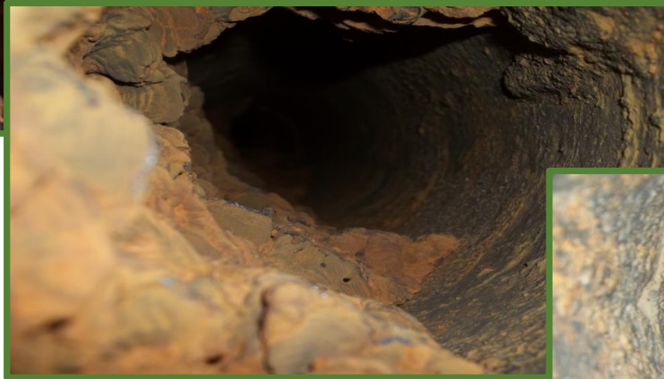
Partial tuberculation removal
