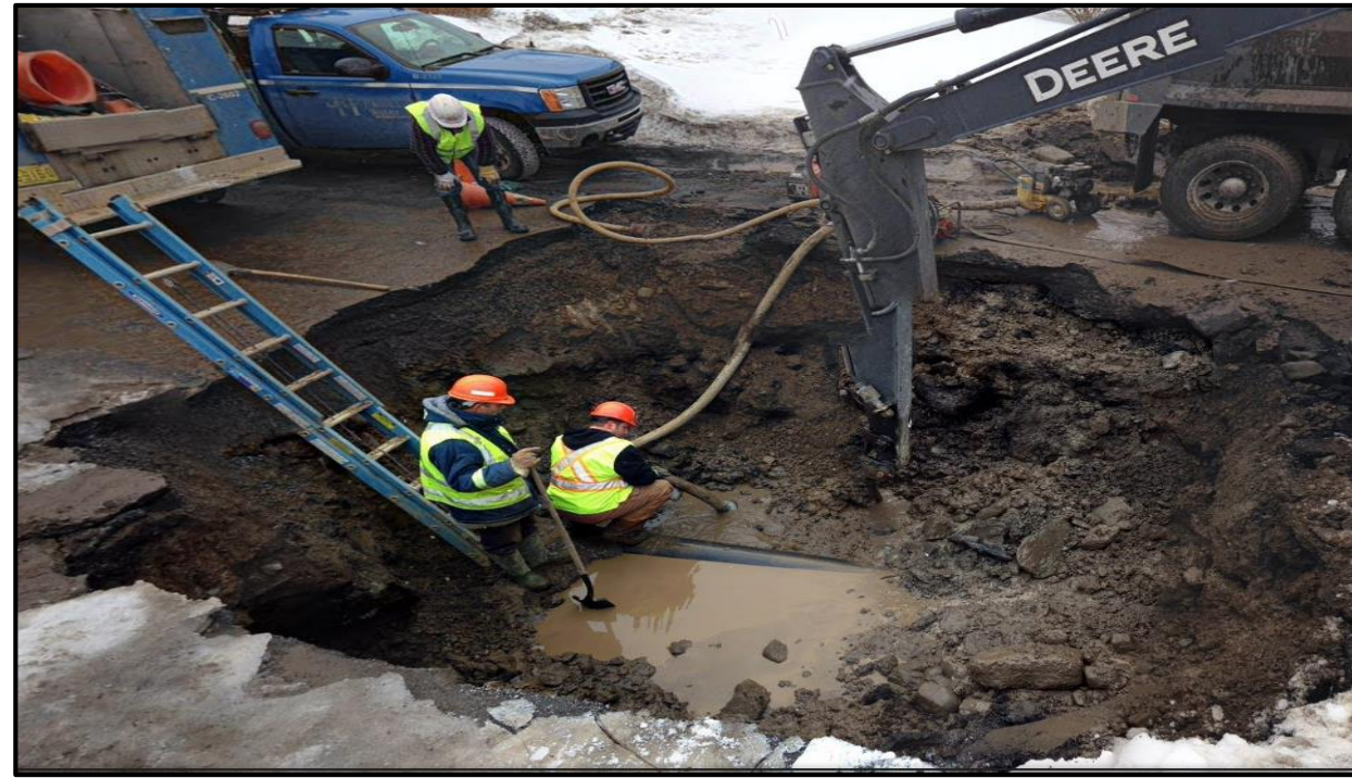
Water main break and repair. Source: Google Maps
