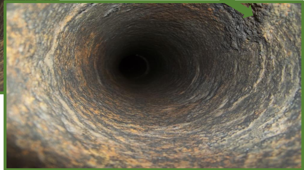
Full tuberculation removal, bitumen liner visible
