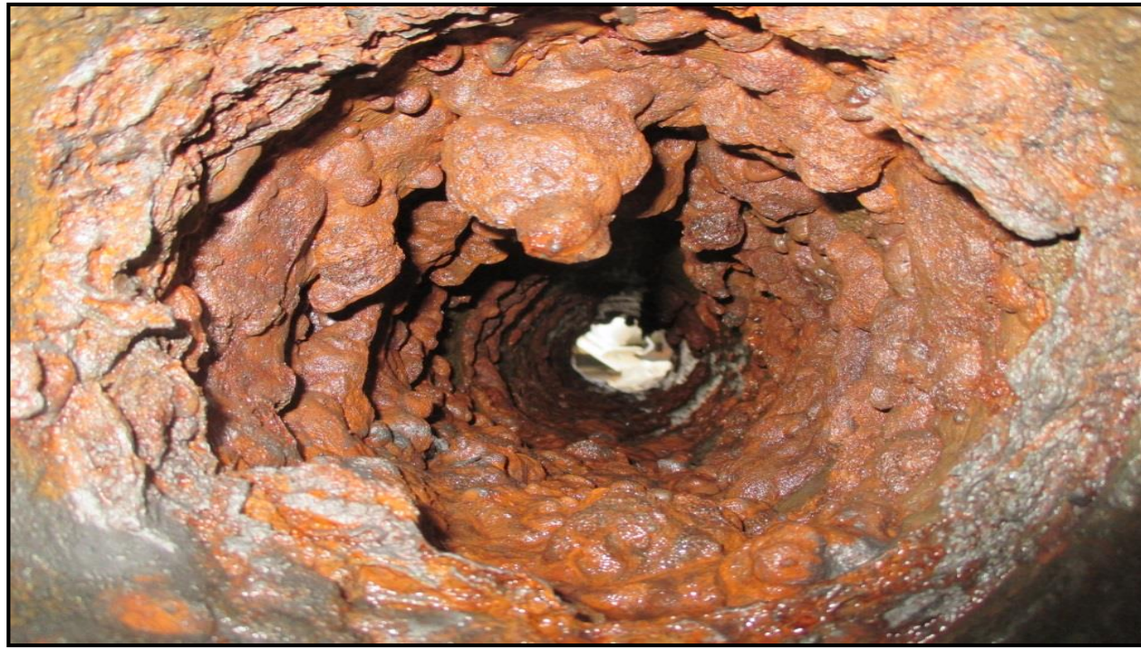
6" tuberculated water main. Photo by Envirolitics
